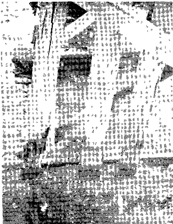
Plate 2. Showing failure of the east outside batter pile of an original full-pile bent because of decay; also shows longitudinal split.
